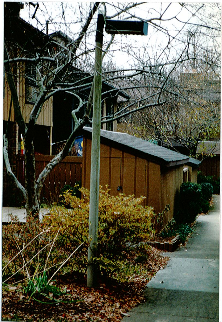
LIGHT POLE Cluster Common Area Shoebox fixture on metal pole (no other specs. on file)
